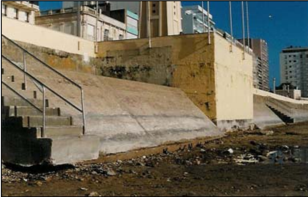
Fig. 4: Before the installation of the beach drainage system, the erosion of the beach caused some damages to the foundations of the seawall.
