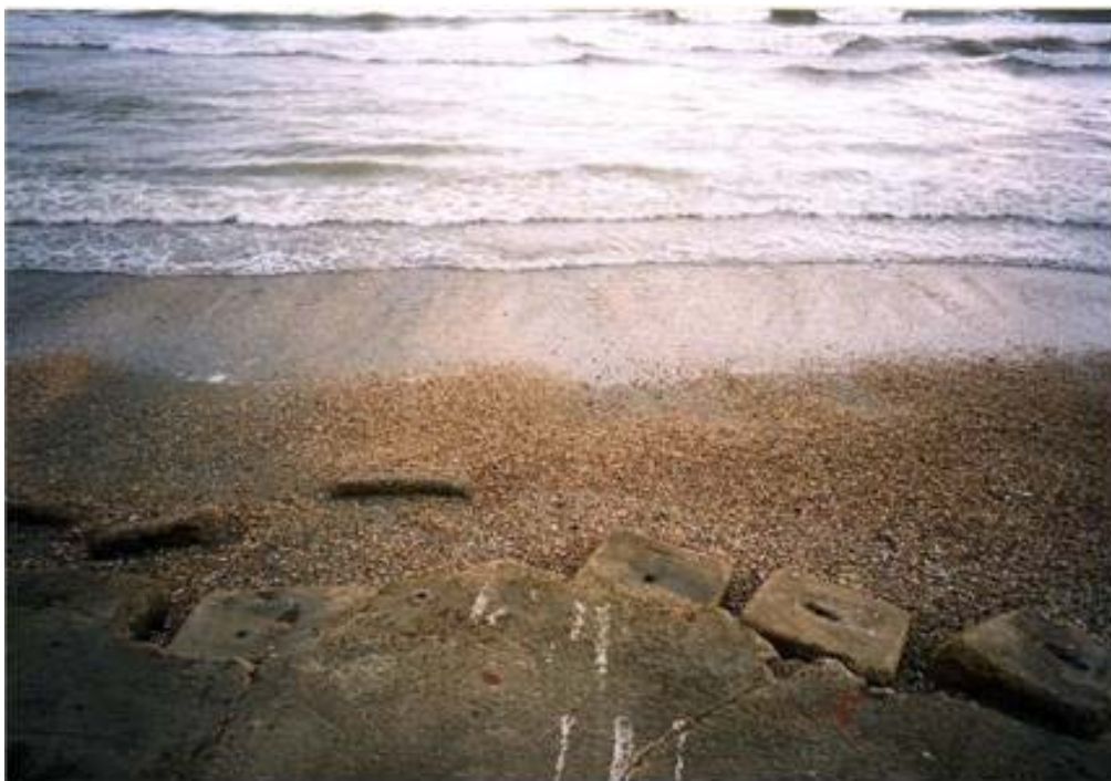
Fig. 6: Example of remains of old passive protection interventions.
